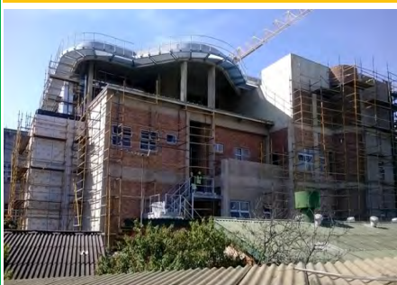
Stanger Hospital gets a facelift state of art maternity and Neonatal Unit READ MORE ON PAGE 2
