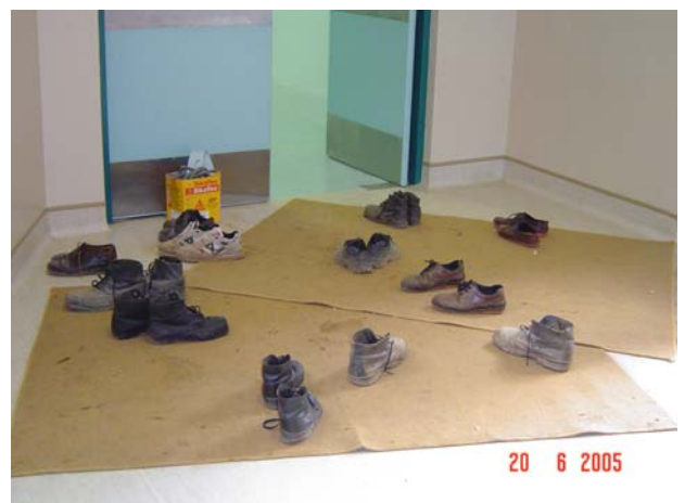
The entrance to the oncology department when the floors were being laid.
