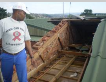
Mr. Leon Andrews (maintenance Section) taken here estimating the damage
