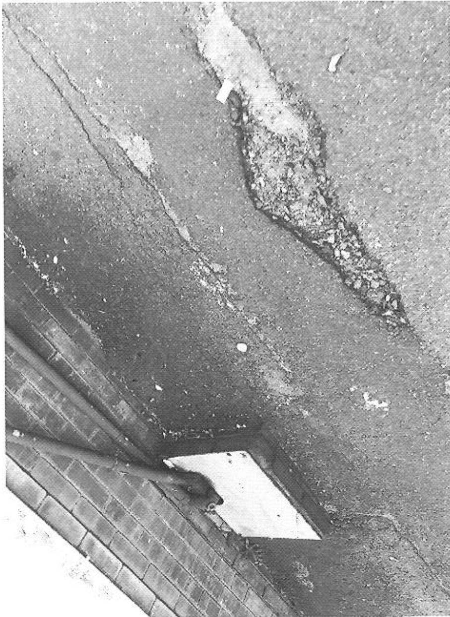
Pothole towards old social work building, pass gate 5.
