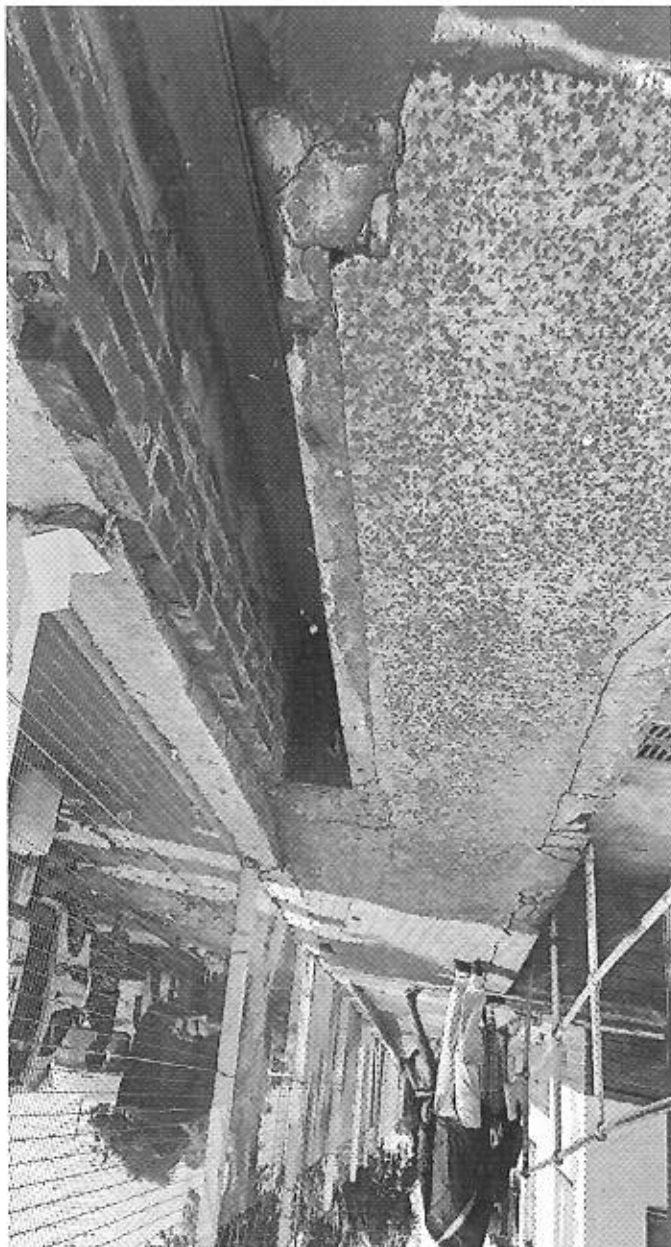
Safety hazard-Missing handrail opposite Rick Turner road (Flu clinic main entrance)
