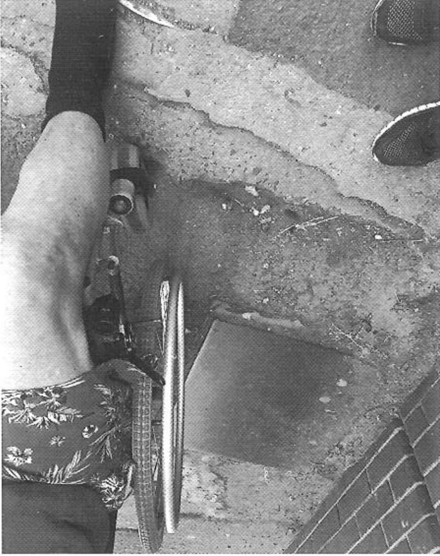
Pothole no.2-Patient struggling to push wheelchair (Between pharmacy and Gate 5)
