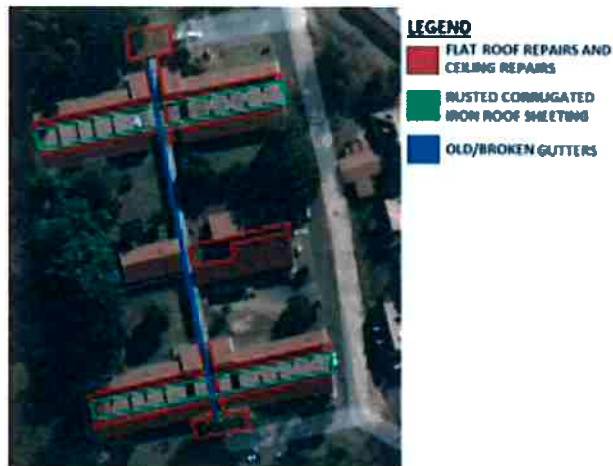
Figure 4-2: Site findings at the Uitsig building
