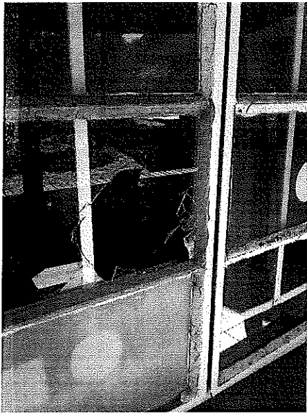
Block A- broken windows
