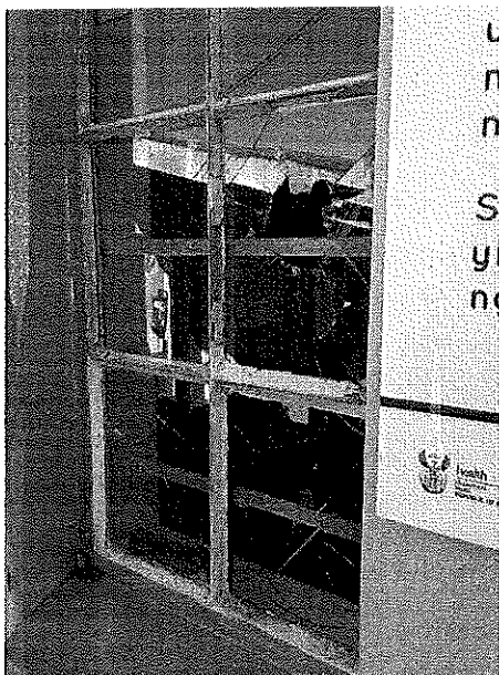
Block A- broken windows at side
