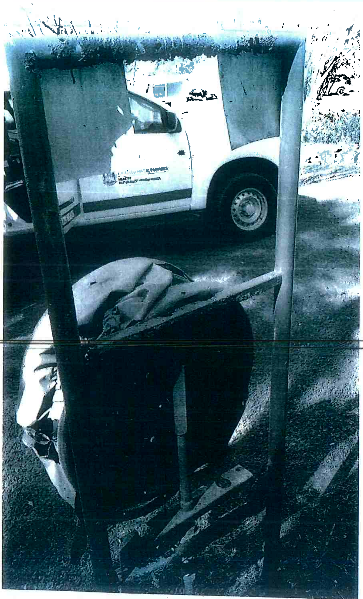
FIRE HOSE REEL STAND,
