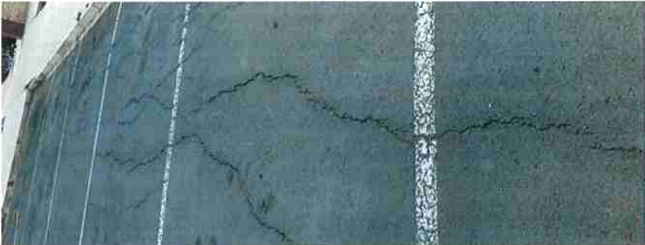
Figure 9 - An example of some of the more severe cracks in the tarred road/ parking surfaces
