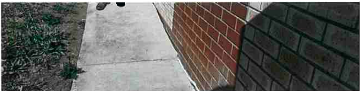
Figure 7 - Apron east of the main complex showing the embankment falling towards the apron without proper drainage. Also note the gap between the wall and the apron in which rainwater that is driven onto the walls infiltrates the substrate
