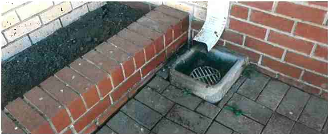
Figure 11 - Courtyard flower box against the building and drain which is not working correctly
