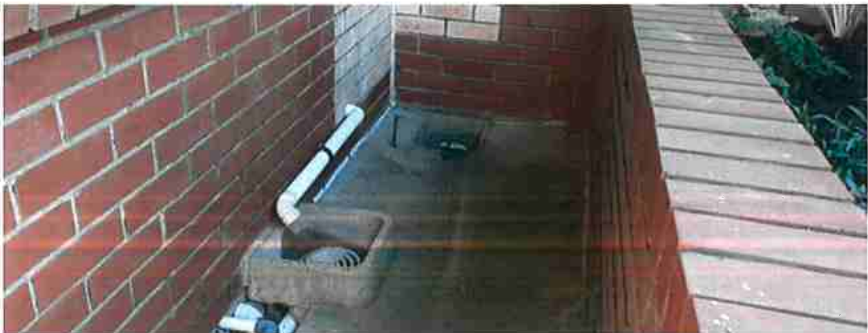
Figure 12 - Courtyard drainage showing drainage and in lower left services which penetrate the surfacing
