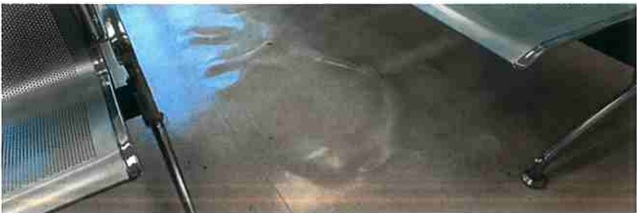
Figure 13 - Damage to the floor covering in a number of wards
