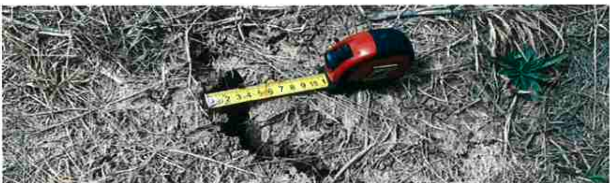
Figure 10 - Desiccation cracking in soil adjacent to the additional administration building There are similar cracks on the east and south sides of the main buildings
