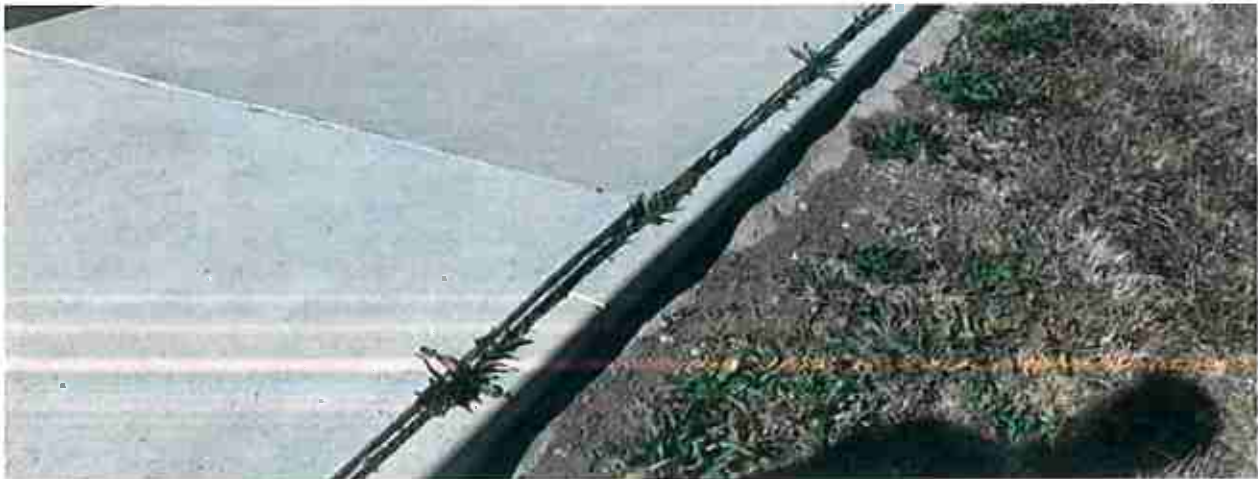
Figure 8 - Typical walkway showing vertical movement between panels and also the kerbs
