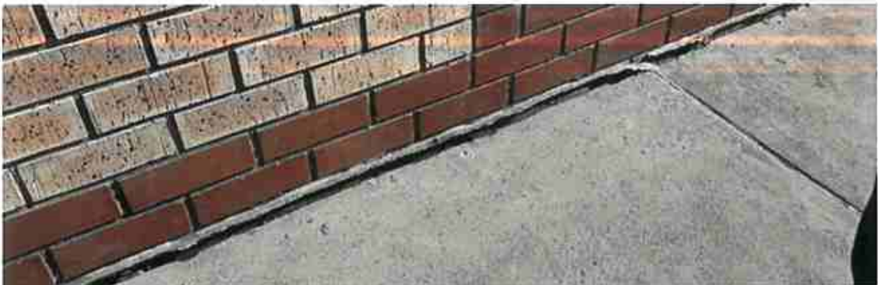
Figure 6 - Gap of over 30 mm between the apron and wall and drop of 25mm in the apron
