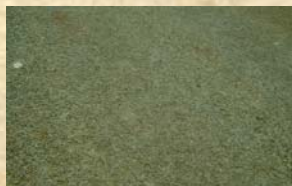
Road surface currently
