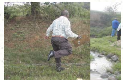
Systems manager Mr. Hlongwane and CEO Mr. Mazibuko taking rounds around the hospital to check the broken fence
