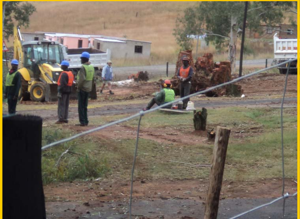
CONSTRUCTION WORKERS ON SITE: NEW OPD STARTING TO TAKE SHAPE, INDEED INCONVINIENCE FOR A GOOD CAUSE
