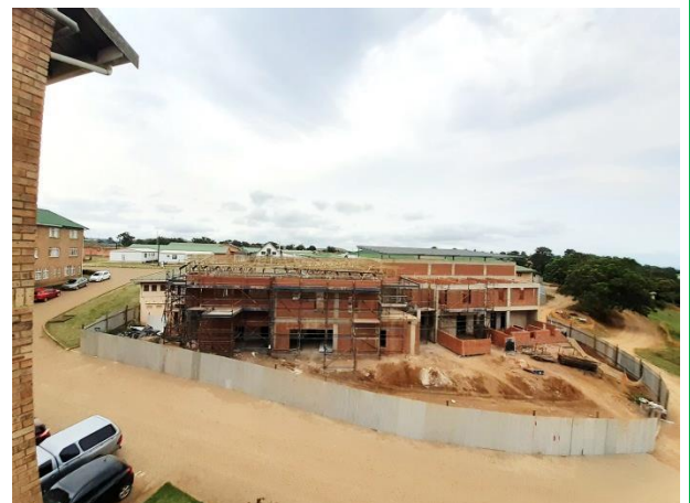
New OPD Still under construction but the complete image gets clearer day by day
