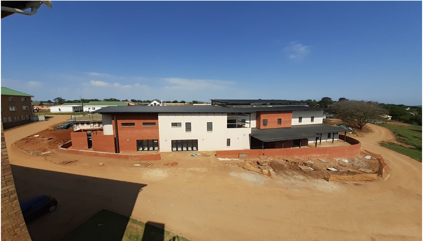
Front view of the new OPD (Reception) that is still under construction. If there was no covid-19 this building was to be done now.
