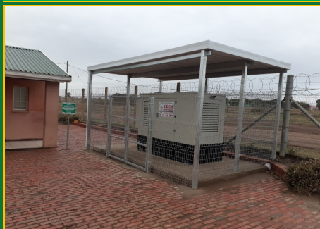
backup generators installation in all clinics ensures continuity of Service.
