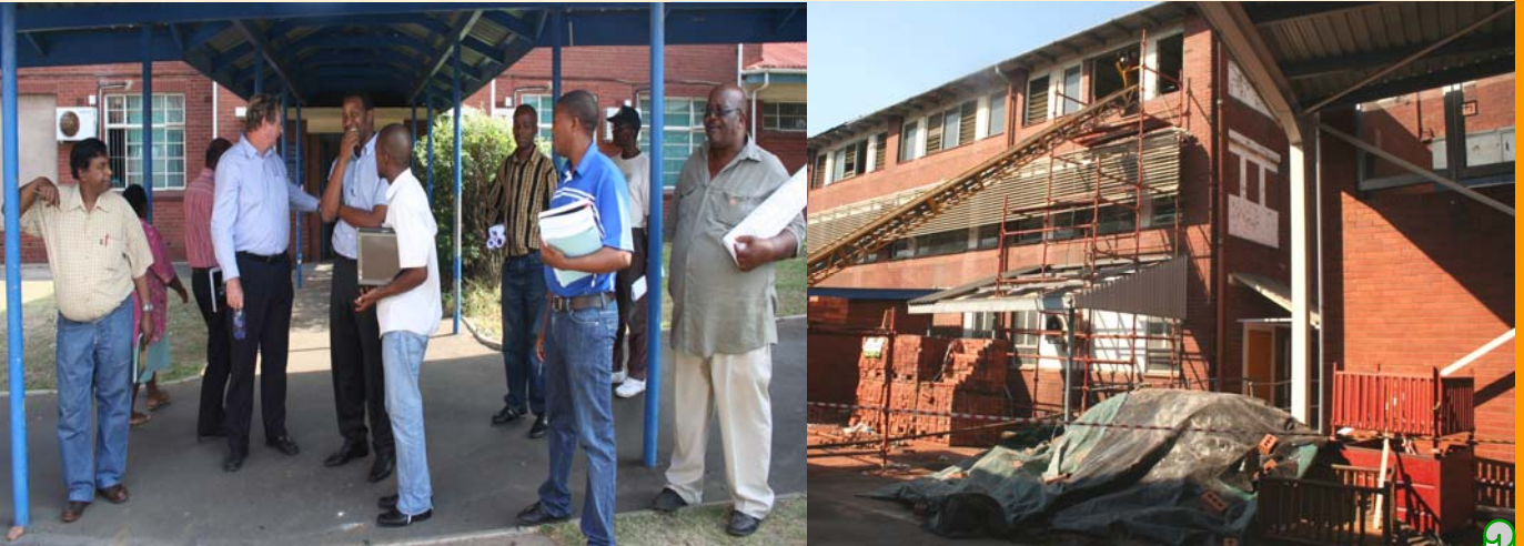
Above: Local and Provincial Team doing a walk about with the contractor before the renovations started. Left: I Block renovations on progress while below N Block roof is erected.
