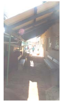
Above: a new shelter connecting the Outpatient and the pharmacy ensuring sheltered walkway.
