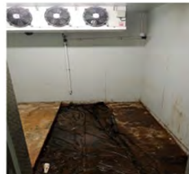
BEFORE, THIS IS HOW COLD ROOM FLOOR USED TO LOOK
